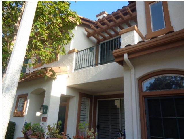
There are typical metal rain gutters and downspouts located throughout the community.
